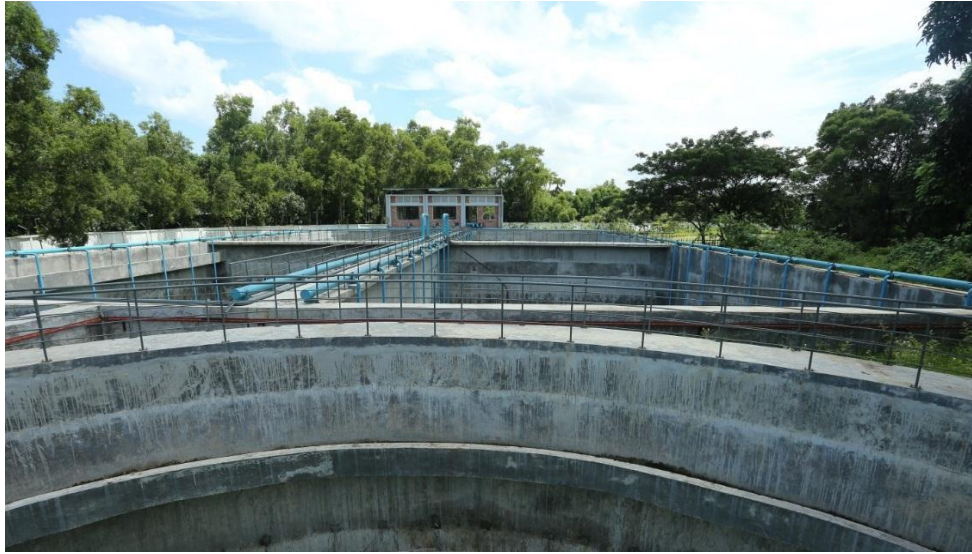
Figure: Complete Biological Effluent Treatment Plant 250 m 3 / hr
